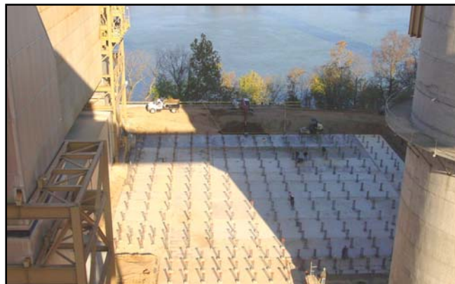
Kentucky Utilities Co. Ghent Generating Station
