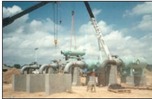
Williams Pipeline - Calvert City Separator
