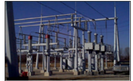
Louisville Gas & Electric - Substation
